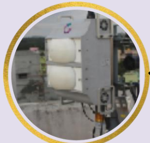
Gigamesh installed at Nidavanda Village
