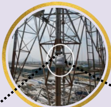
Gigamesh installed on BSNL Tower at Sompura Gram Panchayat
